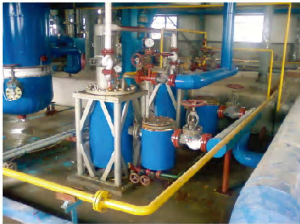
制冷剂项目 氟化氢输送泵 Pump for Hydrogen fluoride in Refrigerant project
