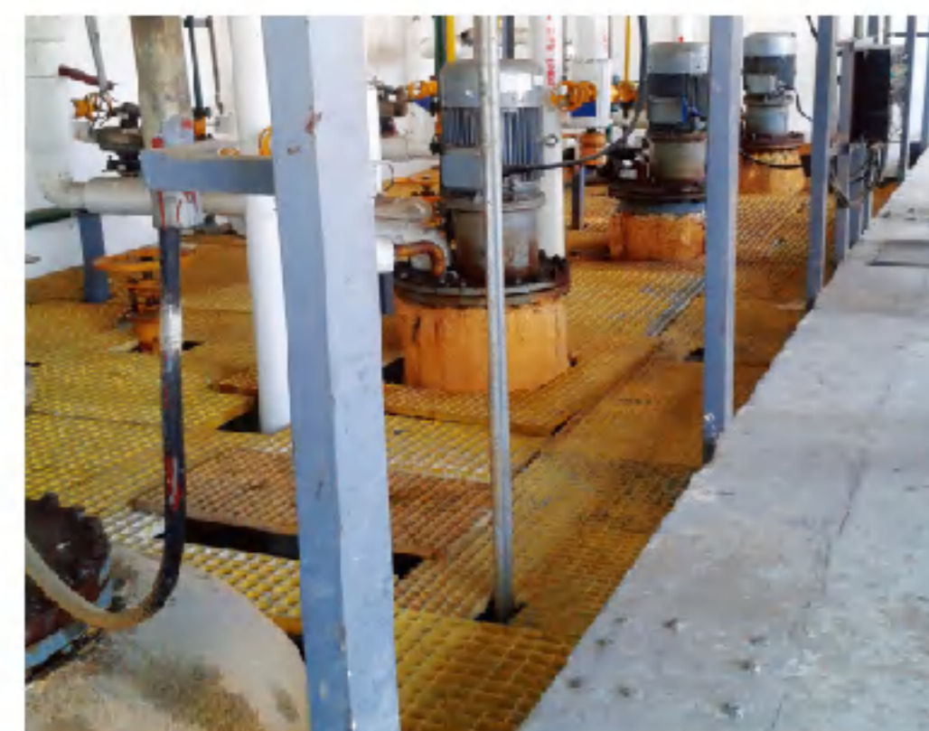
液氯输送泵 Pump for Liquid chlorine 流量Q : 50m 3 /h
