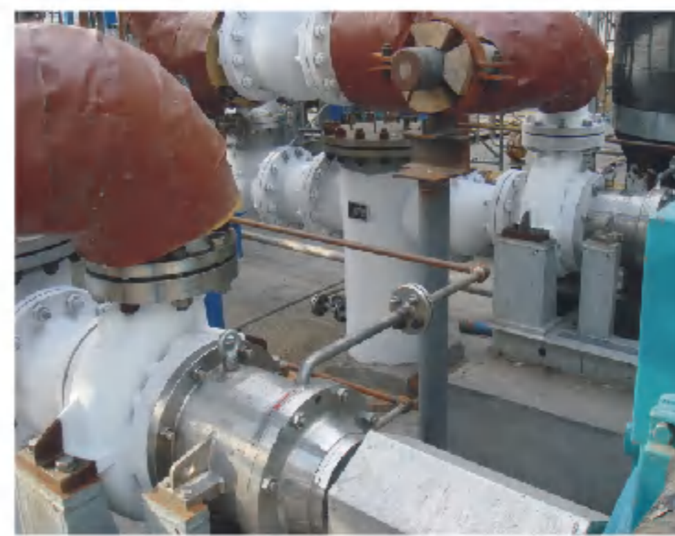
丙烯腈项目 氢氰酸输送泵 Pump for hydrocyanic acid in Acrylonitrile Project
